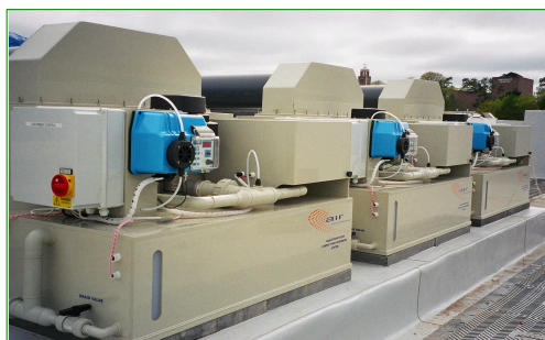
Remote Roof Mounted Scrubbers
